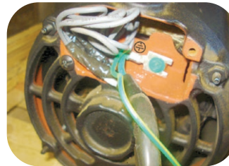
Grounding point in the engine.
