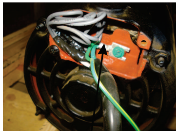
Figure B – Earth point for electric motor
