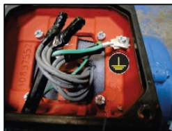
Motor grounding point
