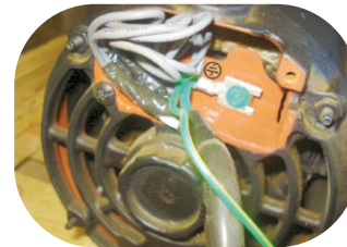
Ground point existing engine.
